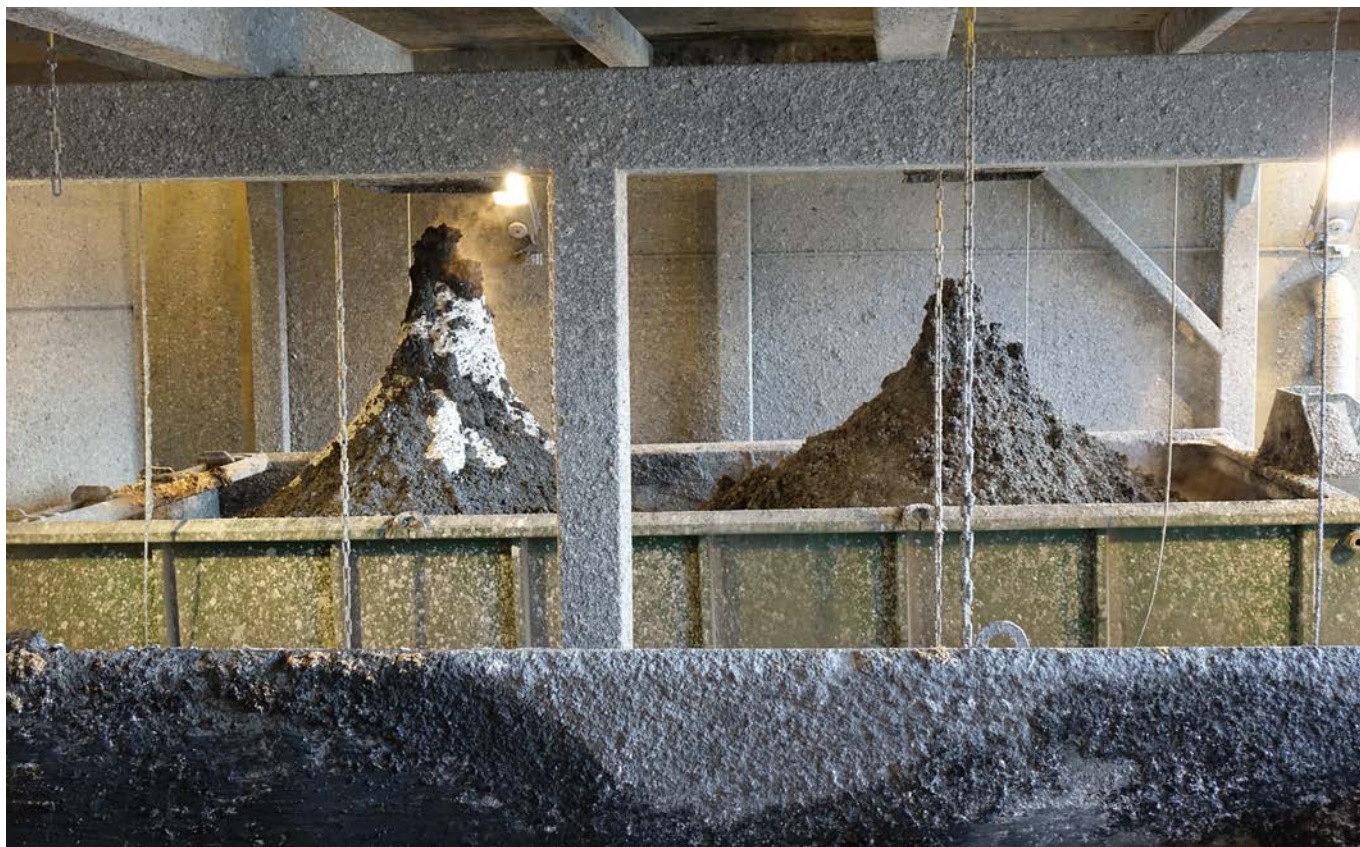
The unloading bay for green liquor dregs at the causticizing plant. Green liquor dregs taken to landfill are loaded onto a flatbed lorry. Photo: Jussi Heinonen.
