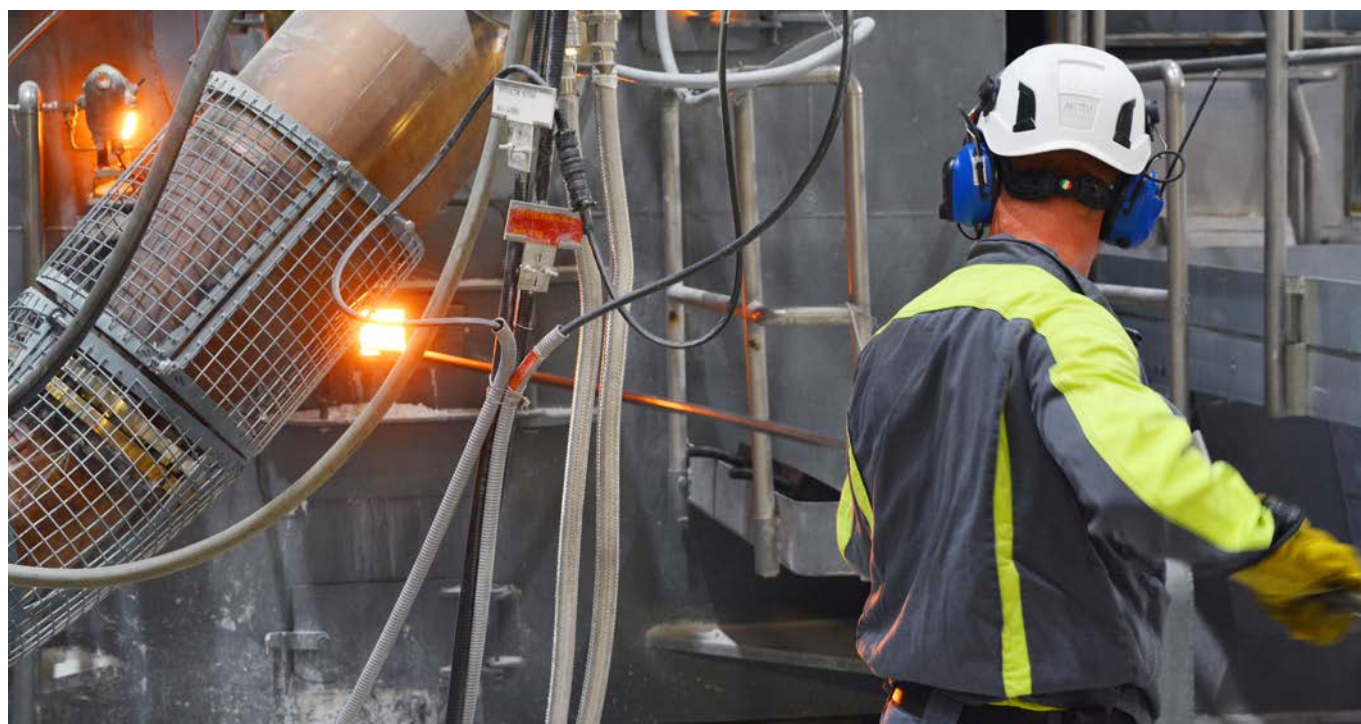
Optimising the operation of the lime kiln is one the pulp mill's objectives for 2020. Photo: Ossi Nikki.
